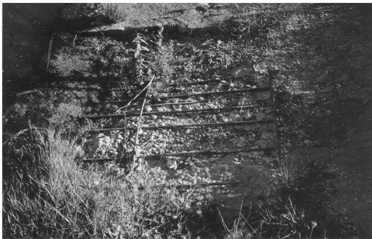
Fig. 3. Erosion of surface on concrete slabs by influence of frost cycles
